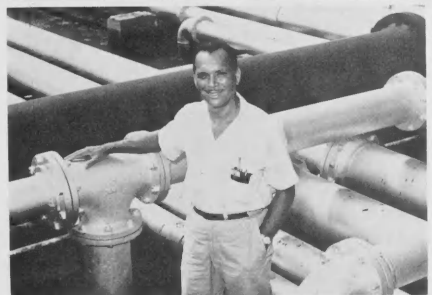
SUGGESTER-OF-the-month is Anselmo Tackling, Process-LOF operator, who suggested the tie-in of a blending line and gas oil transfer from tank to tank 24. The tie-in enables additional pumps to pump from one tank to another. A supplemental award of Fls. 250 was awarded to Mr. Tackling. SUGERIDOR DI luna ta Anselmo Tackling, un operador di Process-LOF, kende a manda un idea pa un coneccion den un linja di blending y cambio di gas oil noord di tanki 24. E coneccion ta permiti pa pompan adicional pomp for di un tanki pa otro. Un premio suplemental di Fls. 250 a worde pagá na Sr. Tackling.
